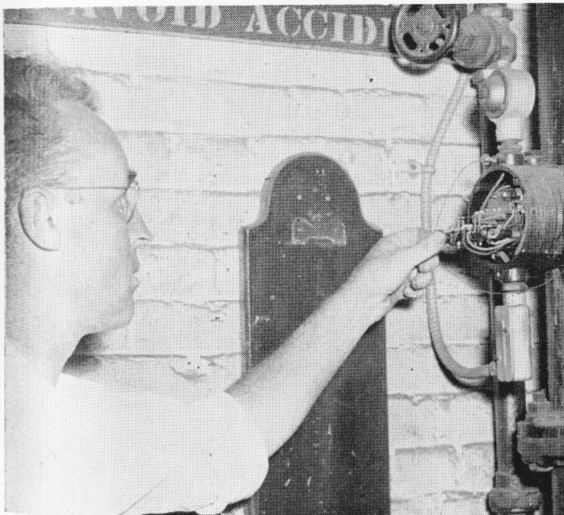
Elmer Crowley watches the sprinkler system. Every week a test of the water flow detectors is made so that at all times a big volume of water will be assured for any blaze rash enough to show its ugly head in any corner around these diggings. Sprinklers are gadgets which pour water over a room when the temperature rises above a certain point. They're always faithfully on the job.
