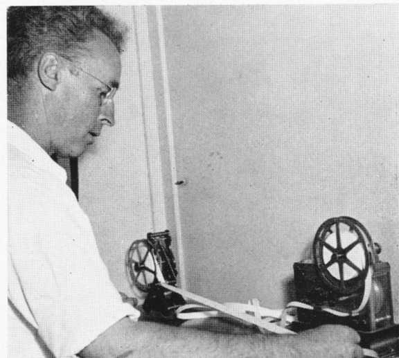
The Signal system of the plant is tested several times daily, and the signals must record correctly on signal lamps and, in the case of fire, on ticker tapes, all of which are located in the telephone switchboard room. All in all it is apparent that the Signal and Call girls and boys are watching over us pretty carefully to see that no disaster comes to us. They seem to be our central nervous system.
